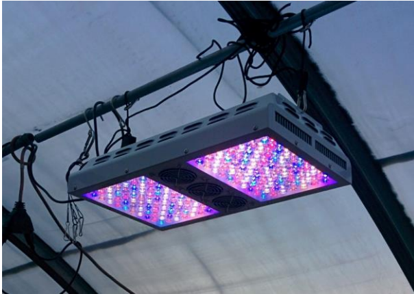
Plate 93. High lighting critical for successful glasshouse sweetpotato studies.
